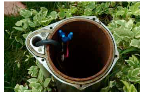
Brendan notes the well's pipe is clean and in good order but identifies that waterproof connectors were not used for the pump's electrical connection.
