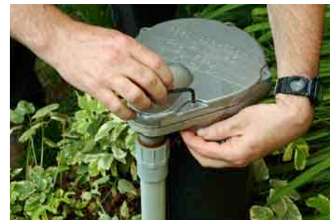
Brendan shows Albert how to remove the well cover, to check the condition of inside of the pipe.
