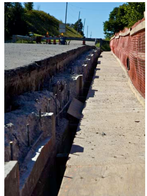
This photo, taken in late August, shows the extent of the reconstruction underway to restore the handrails on the Siegner Bridge near Kingwood. Ninety percent of the work on the bridge is now complete, relying on alternate funding until the government funding arrives.
